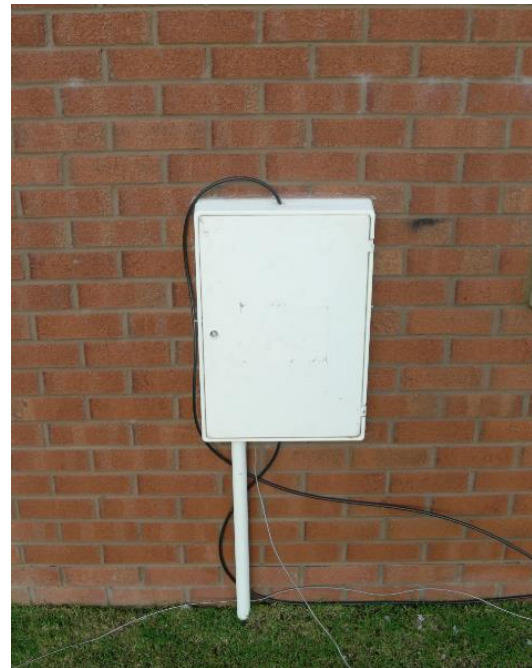
Figure 8: External meter box (2)
