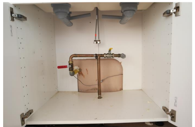
Figure 19: Under sink cupboard
