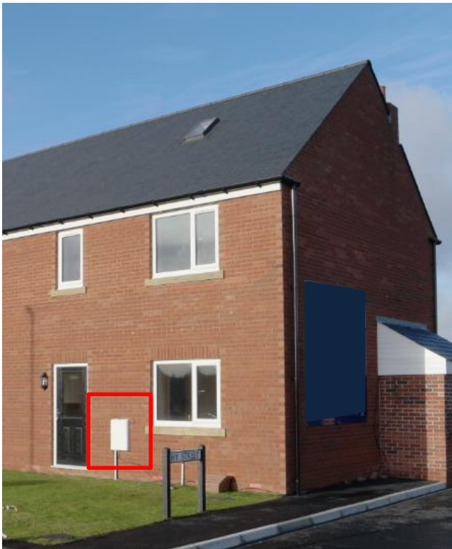
Figure 7: External meter box (1)
