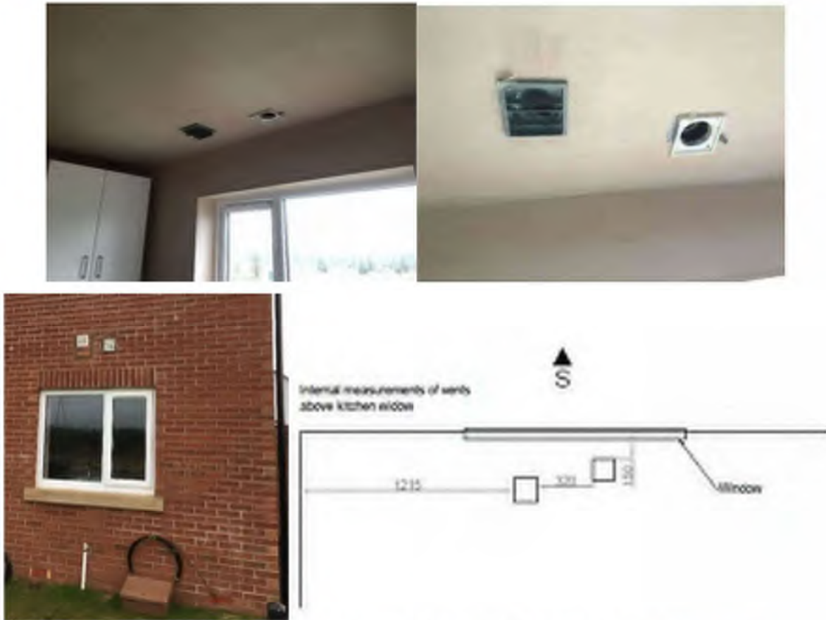
Figure 11: 78 cm 2 and 141 cm 2 ducted ceiling vents in kitchen
