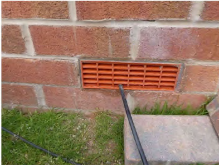
Figure 12: 65 cm 2 opening air brick into basement c/w sample line inserted
