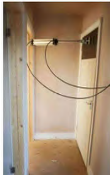
Figure 15: Pneumatic ram operating basement door
