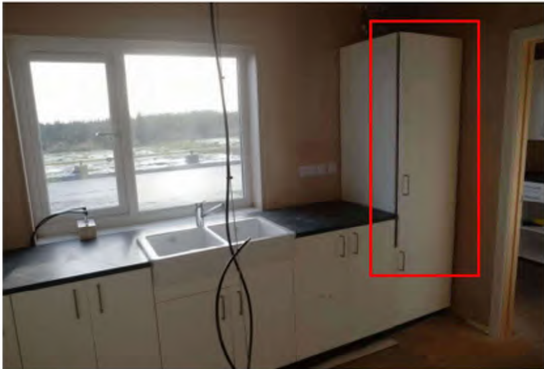
Figure 3: Location of boiler cupboard in kitchen
