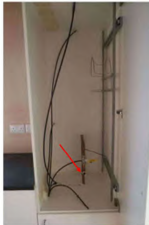
Figure 27: Inside boiler cupboard (arrow indicates release point)
