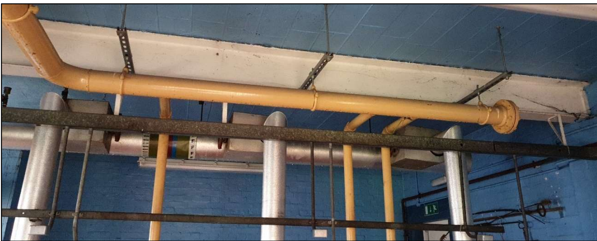
Figure 7: 4-inch gas pipework showing end plate and 2-inch boiler feed pipes
