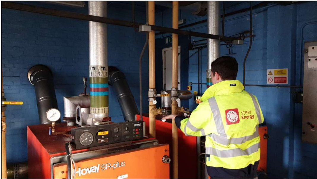
Figure 12: Second and third boilers
