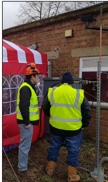
Figure 15: Purge stack with flow volume meter in operation
