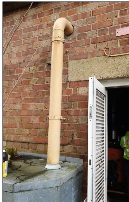
Figure 5: Four-inch pipe from meter cabinet into the plant room
