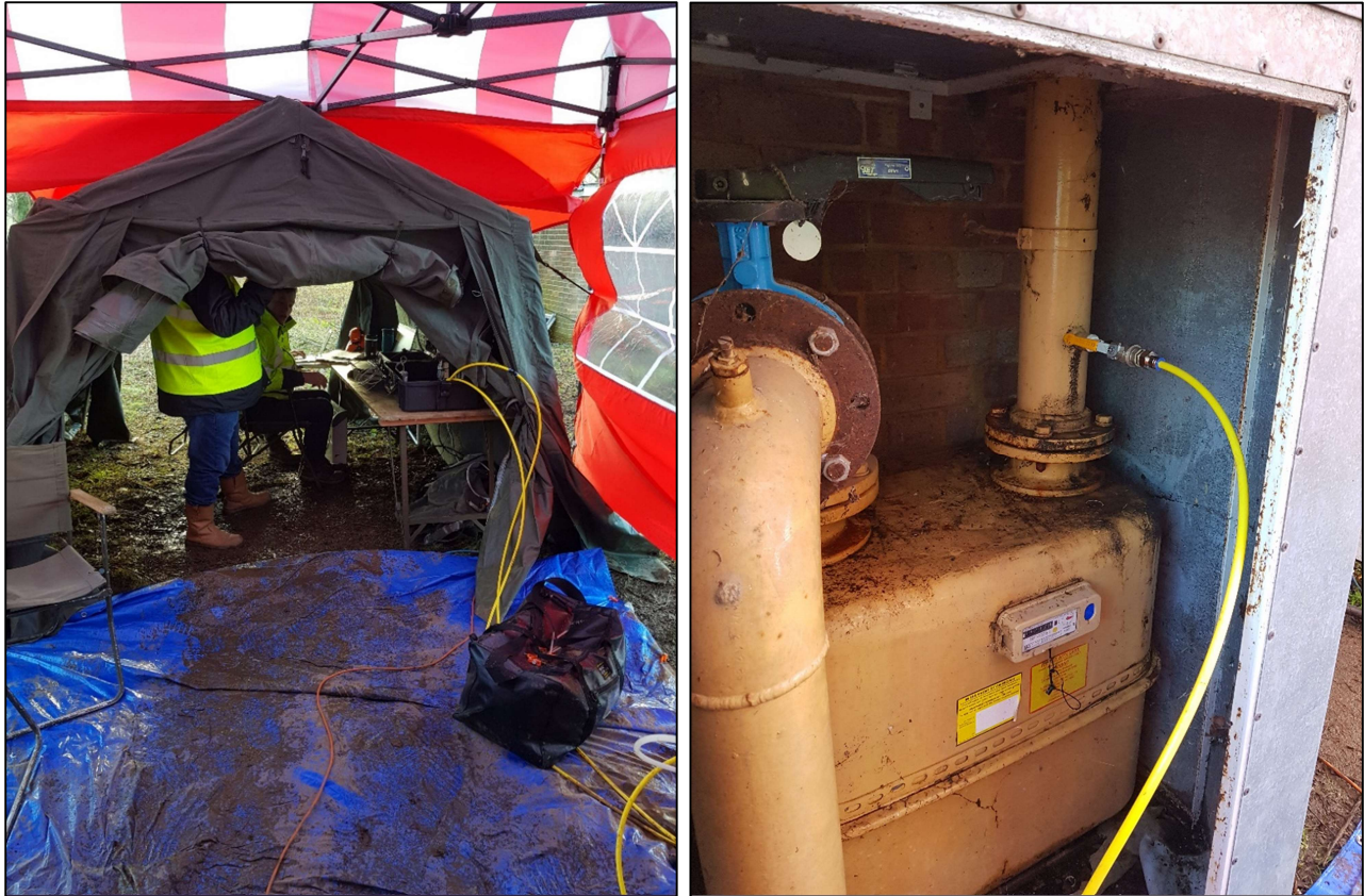
Figure 16: Hose management from test equipment through to gas injection point
