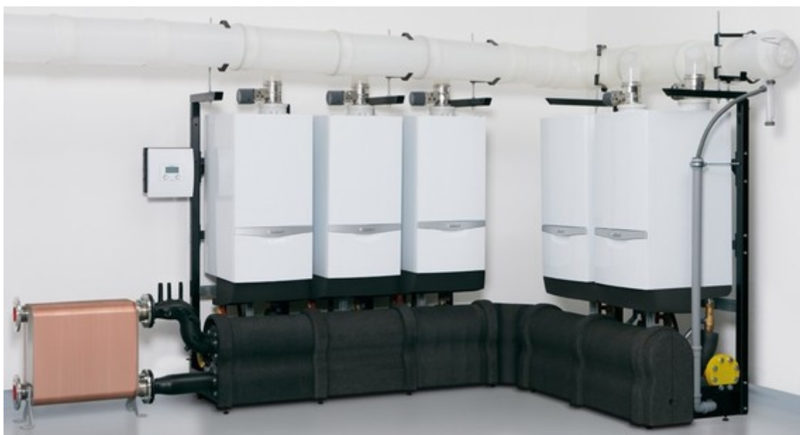
Figure 4-5 – Cascade Boiler System
